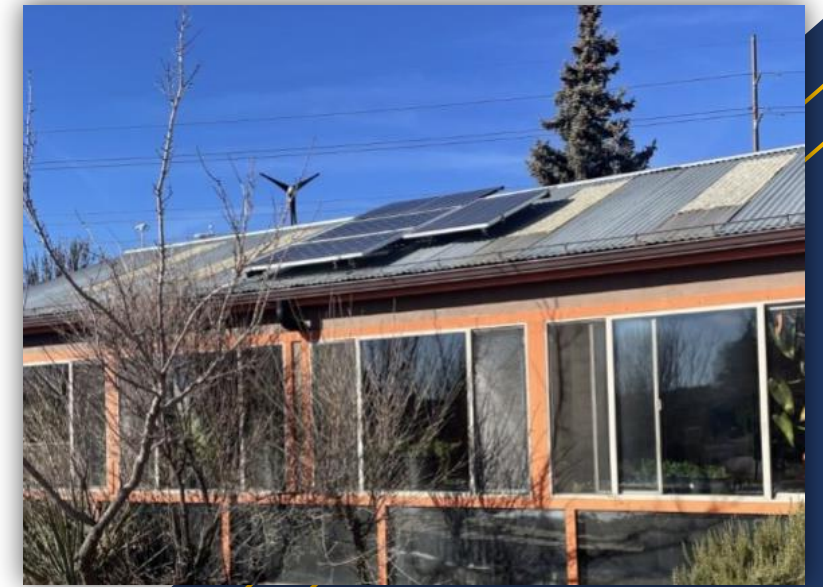
Fig 12. PHS Greenhouse Solar Panels
