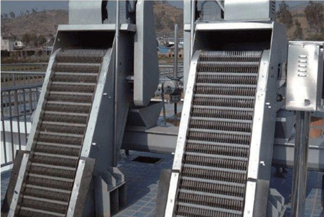
Figure 4: Vertical Bar Screens
