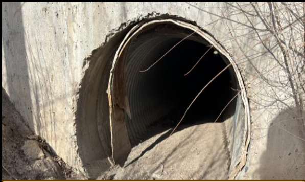
1 Culvert Condition Sediment buildup
