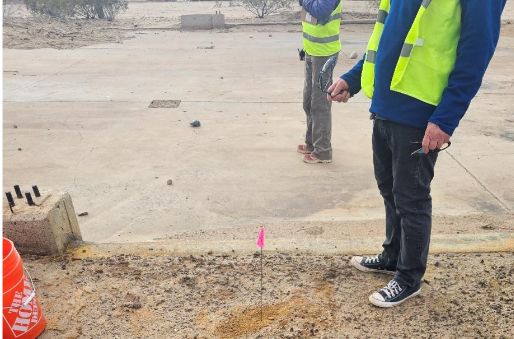
Figure 3.6: Concrete Pad (credit: Rashel DeLeon)
