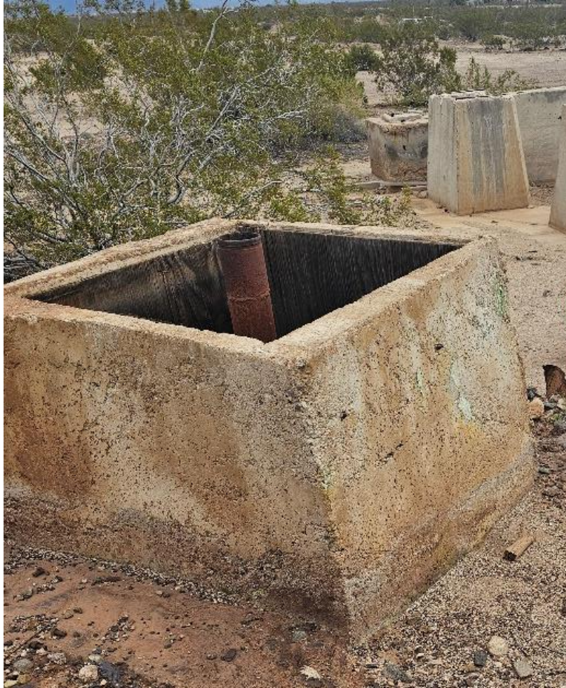
Figure 3.4: Concrete Box and Concrete Pad (credit: Rashel DeLeon)
